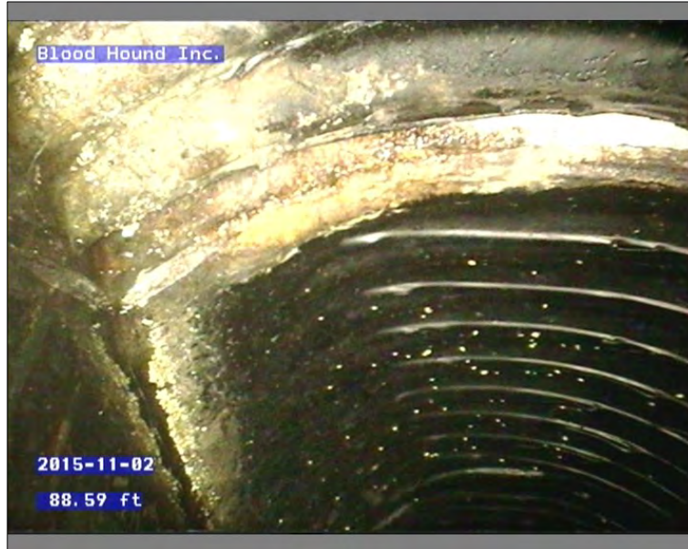
Photo: 45639-110215-01-AECOM-10211201511445711445757_A.JPG, 00:10:56 88.59FT, Surface Reinforcement Corroded, from 07 to 09 o'clock, within 8 inches of joint: YES
