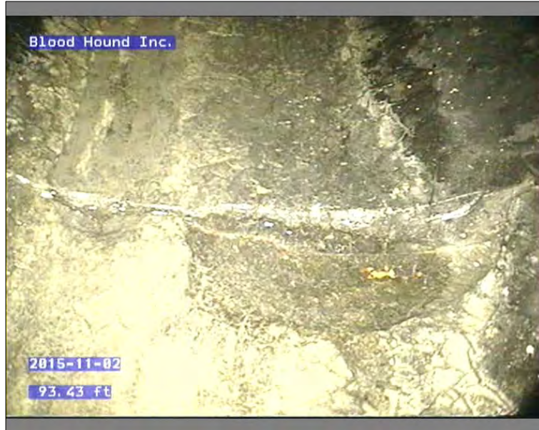
Photo: 45639-110215-01-AECOM-10211201511501311501313_A.JPG, 00:14:55 93.43FT, General Observation
