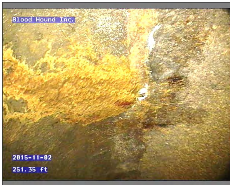
Photo: 45639-110215-01-AECOM-10211201512053112053131_A.JPG, 00:27:51 251.35FT, Surface Reinforcement Corroded, from 06 to 09 o'clock, within 8 inches of joint: YES
