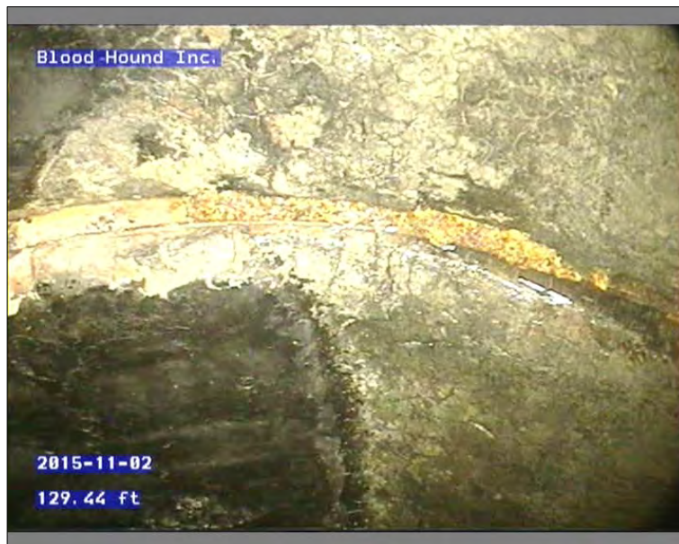
Photo: 45639-110215-01-AECOM-10211201511543211543232_A.JPG, 00:18:27 129.44FT, Surface Reinforcement Corroded, from 03 to 05 o'clock, within 8 inches of joint: YES
