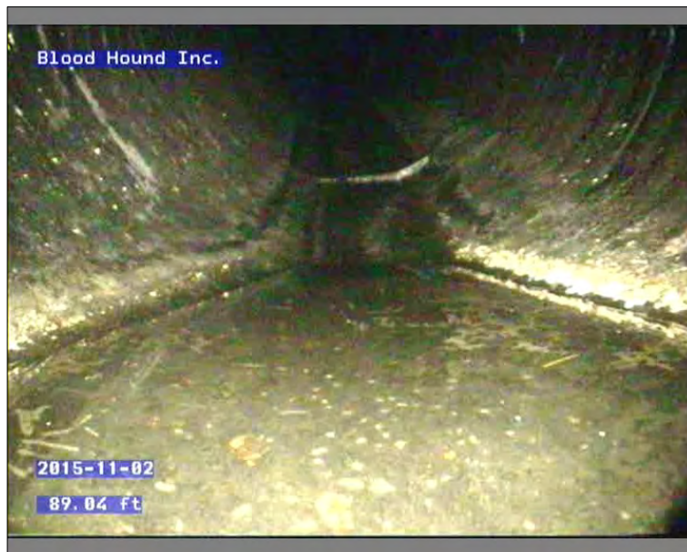
Photo: 45639-110215-01-AECOM-10211201511475311475353_A.JPG, 00:13:05 89.04FT, General Observation
