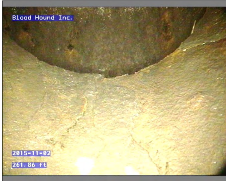
Photo: 45639-110215-01-AECOM-10211201512081712081717_A.JPG, 00:29:27 261.86FT, Surface Roughness Increased, from 05 to 07 o'clock, within 8 inches of joint: YES, Finish
