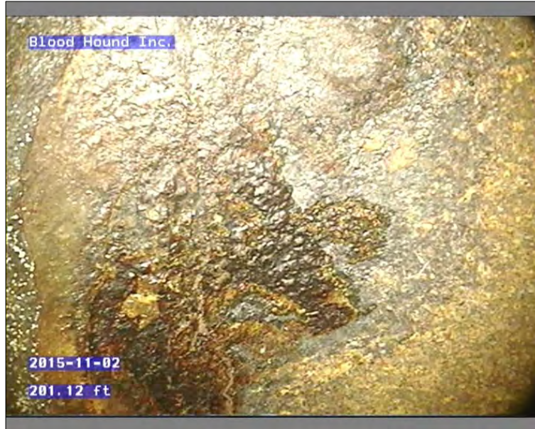
Photo: 45639-110215-01-AECOM-10211201512010812010808_A.JPG, 00:23:59 201.12FT, Infiltration Weeper, at 09 o'clock, within 8 inches of joint: YES
